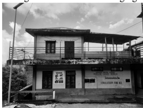
Special School for the Blind building, dorms and classrooms. Photo by Rodingpuii, September 30, 2025
